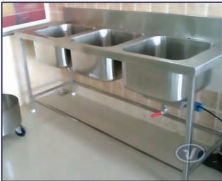
THREE SINK WASHING UNIT
