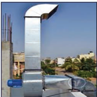
EXHAUST DUCTING SYSTEMS
