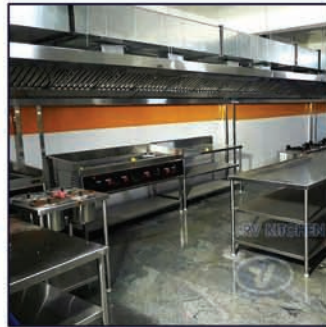
EXHAUST HOOD &/ DUCT
