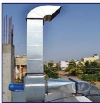
EXHAUST DUCTING SYSTEM
