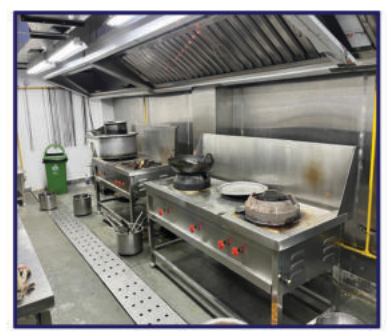
EXHAUST HOOD &/ DUCT
